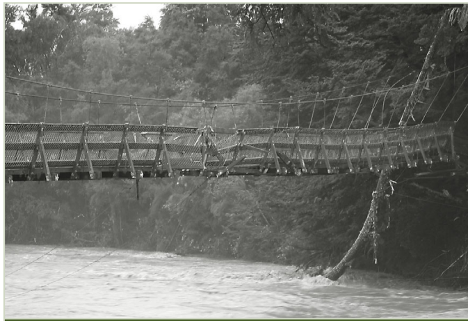
The Major Jones Bridge was badly damaged at the height of the February 2004 flood. It took several frustrating months to repair.
