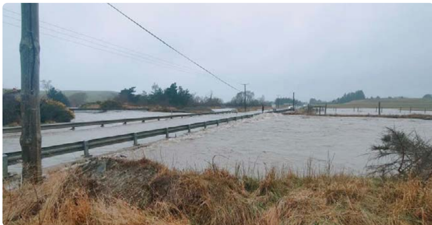
Flooding of Big Kuri Creek closes State Highway 1, just north of Hampden, in Otago, last week.
