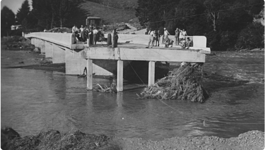
The bridge survived but the abutment from road to bridge was washed away.
