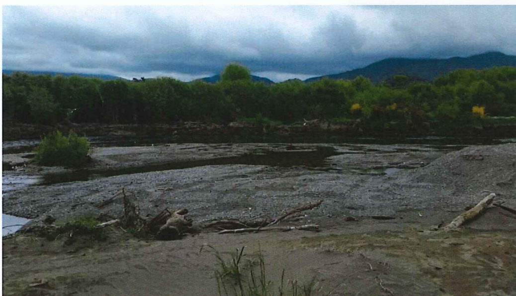
Figure 3-4 Active erosion and overtopping of left bank at Downs Pool and sediment deposition on inside of bend. Note low areas of bank.
