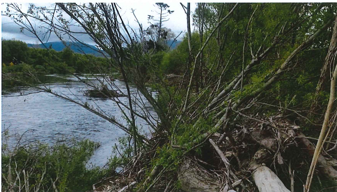
Figure 3-3 Active erosion and overtopping of right bank immediately downstream of De Latours shortcut
